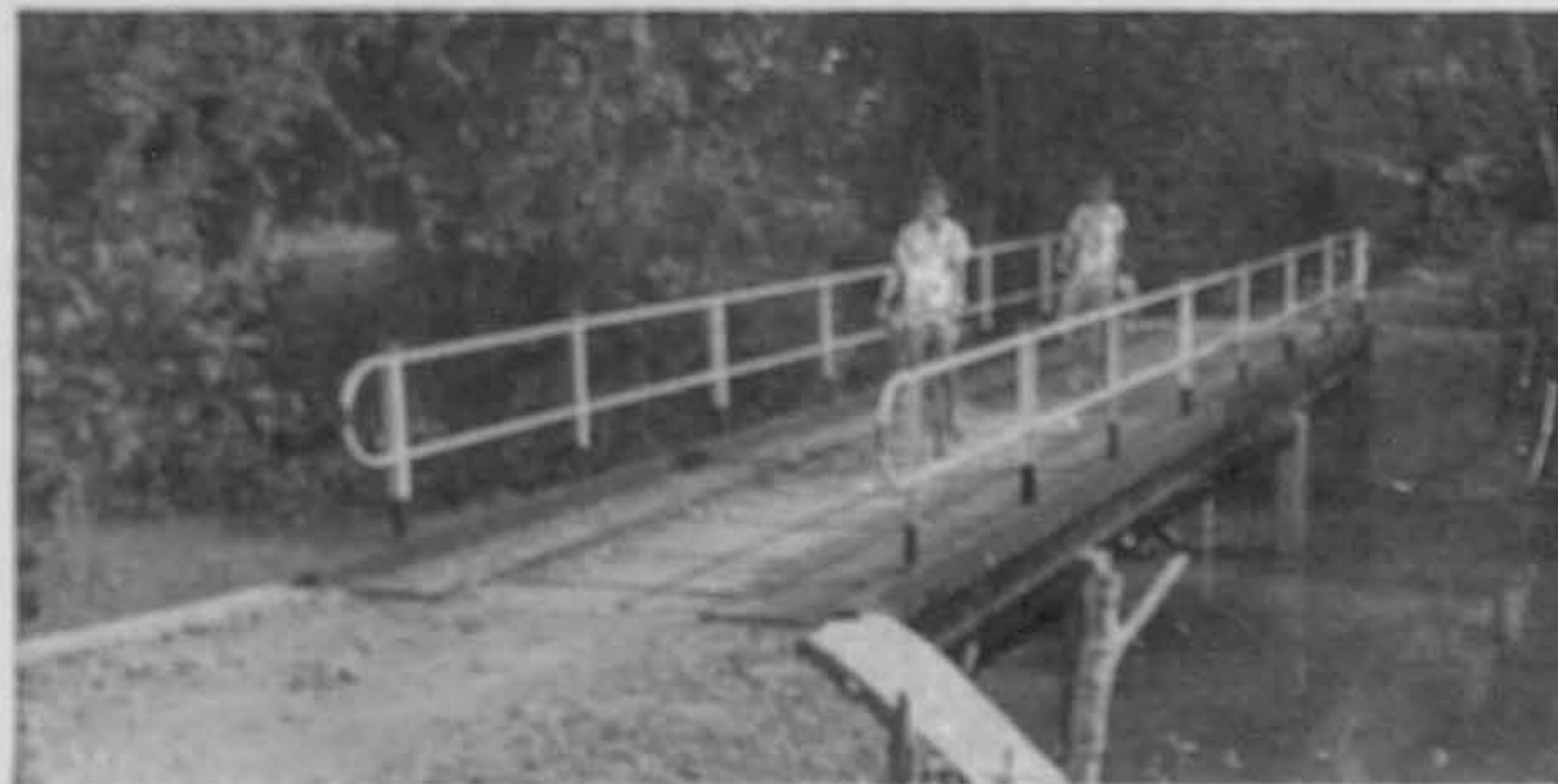
A wooden bridge like this helps the villagers to transport their kampong produce to a nearest town. This bridge at Kampong Alor Raja, in Kedah, was built at the cost of $9,000.
