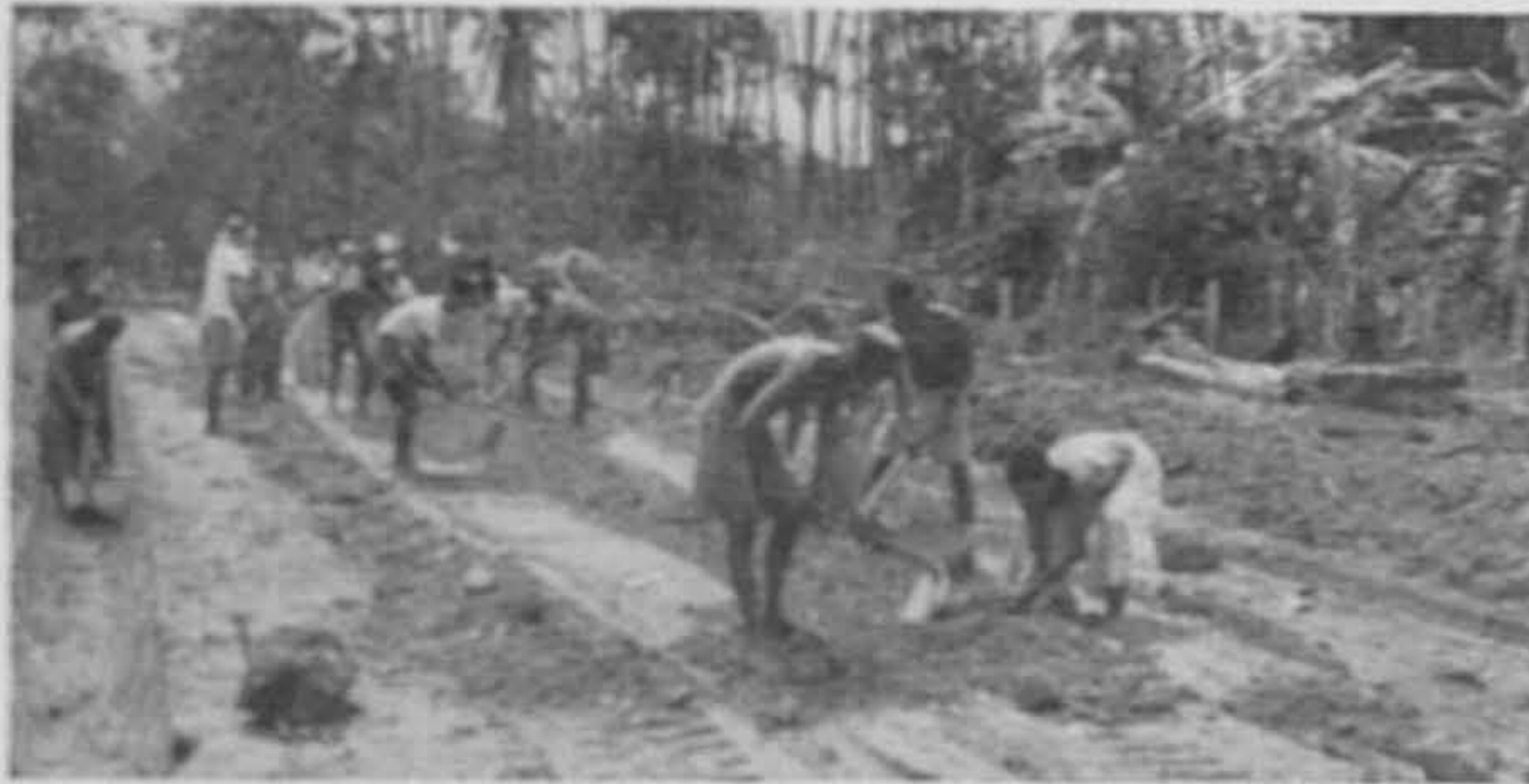
Traditional spirit of co-operation (Gotong Royong) prevails—a 6-mile kampong road to connect Kampong Lukut and Simpang Makam, in Kota Tinggi District, being built by villagers with materials costing $33,000 supplied by the Government.
