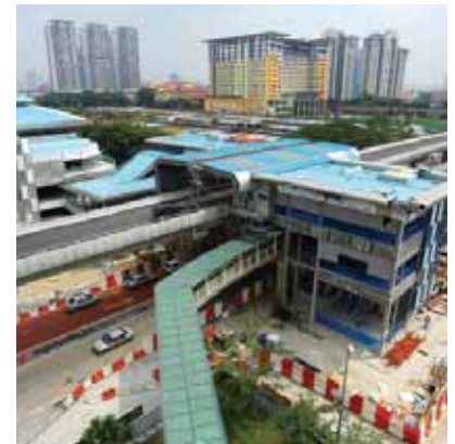
Bus Rapid Transit (BRT) – Sunway Line is under construction and to be launched in June 2015
