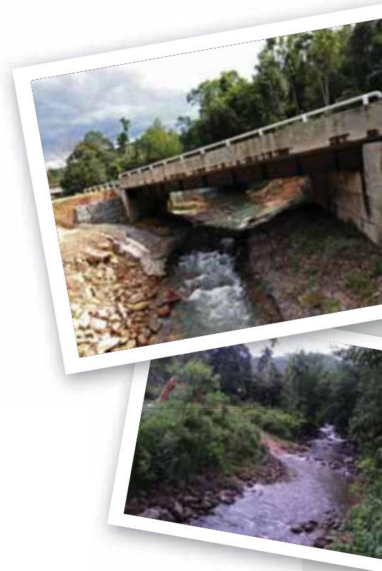
Before and after the roads upgrading project at Jalan Sugud Timpangoh, Penampang, Sabah
