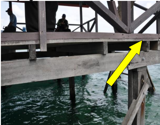
Gambar 2.1 Panjang Beam 2" x 5" Kurang 61.58 Meter
