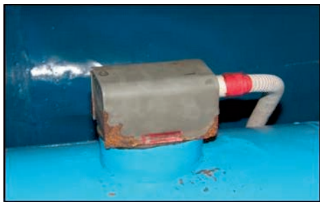
Chiller Plant Room - Penutup Flow Switch Berkarat (16.01.2013)
