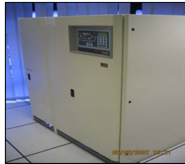
Uninterrupted Power Supply
