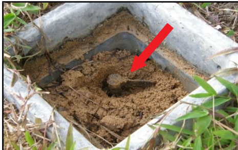
Luar Kompleks - Sistem Pembumian - Tiada Penandaan Label "Safety Electrical Connection - Do Not Remove" Or "Lightning Protection Earth - Do Not Remove" (12.06.2012)
