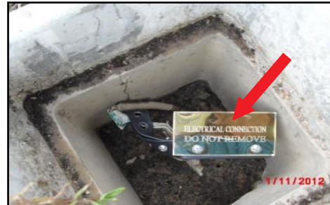
Luar Kompleks - Sistem Pembumian - Penandaan Label "Safety Electrical Connection - Do Not Remove" Or "Lightning Protection Earth - Do Not Remove" Telah Dipasang (01.11.2012)
