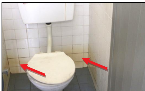
SK Bandar Sunway, Petaling Jaya, Selangor - Dinding Jubin Tandas Berlumut (07.08.2012)
