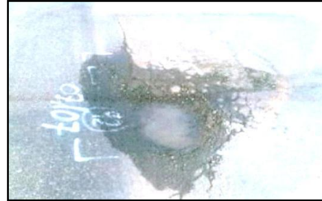
- Pothole Di Taxiway (Sumber: MASB) (27.06.2011)
