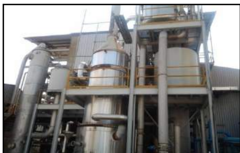
Syarikat Dovechem Chemical, Kuantan, Pahang - Off-Gas Recycle Plant (22.05.2013)
