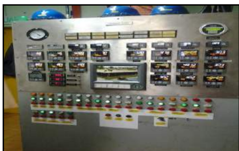
Syarikat Dovechem Chemical, Kuantan, Pahang - Panel Pengawalan Off-Gas2 (22.05.2013)
