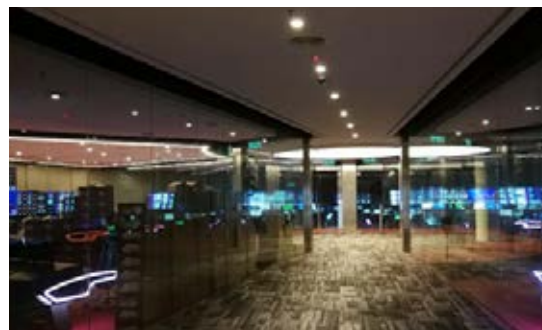
Transmission Operating Centre
