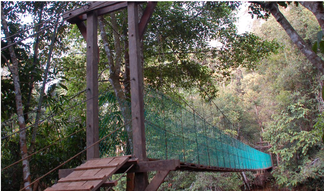
Finish product of 32-metres long suspension bridge across the Kubaan River in Long Semirang, Upper, Baram, Miri, Sarawak Photo by Forest Department Sarawak
