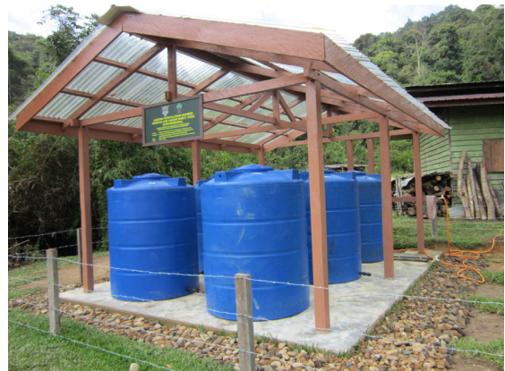
Two photos vertically right - Upgraded hill salt processing facilities Photo by Forest Department Sarawak
