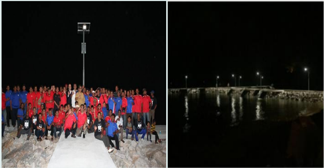
The launch of LED solar street lights at Kampung Hailan Jetty, Tangga Batu, Melaka
