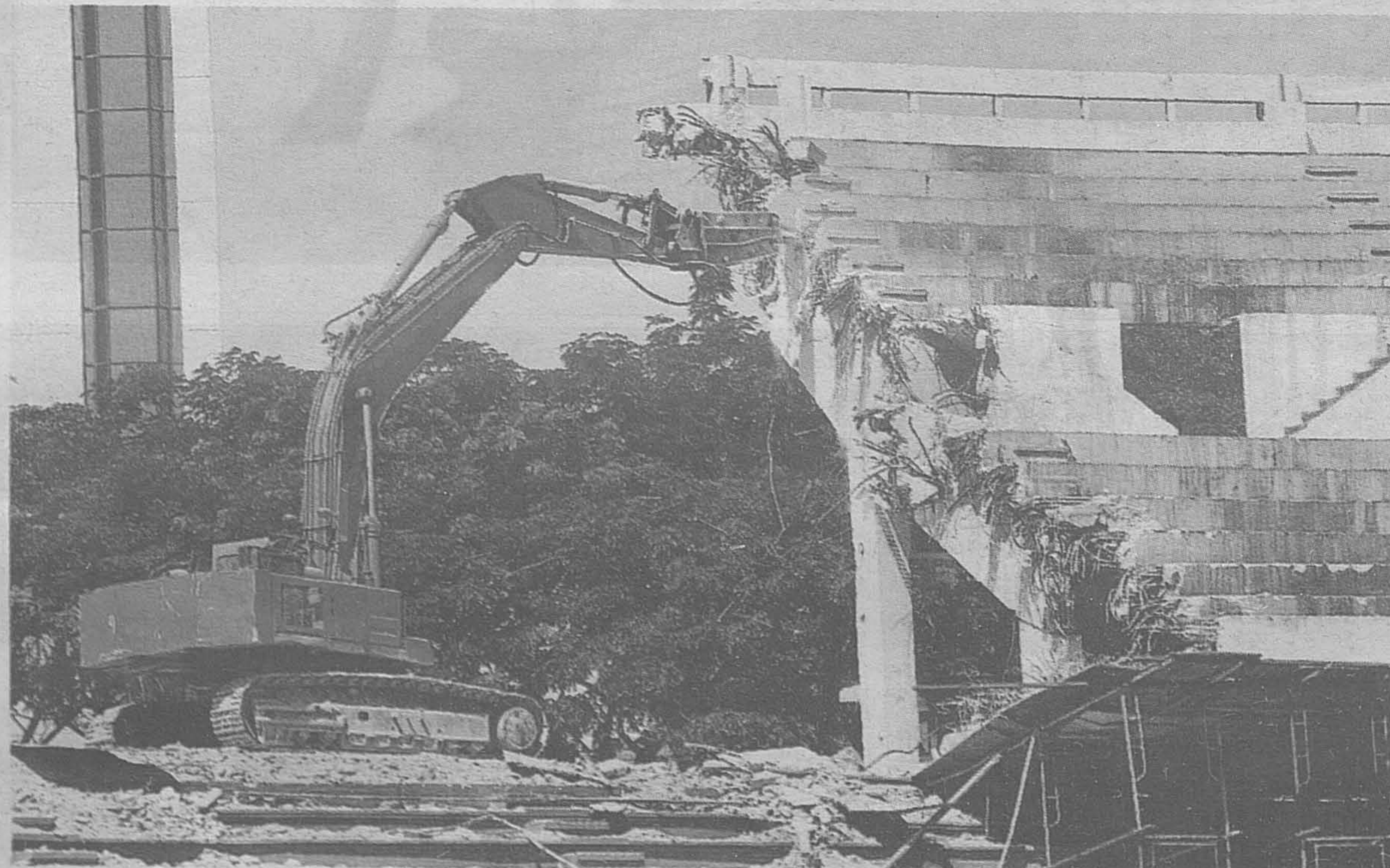
Demolition time: One of the stands being brought down to bring Merdeka Stadium back to its original specifications.
