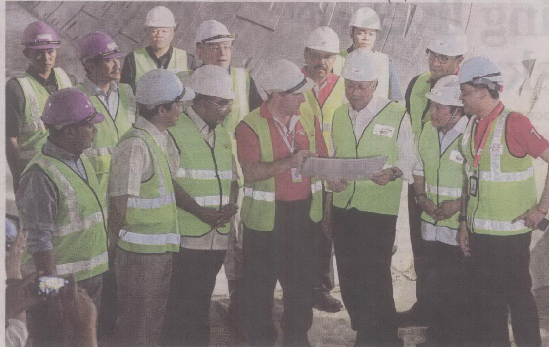
Datuk Seri Najib Razak speaking to SBK route project manager Marcus Karakashian (fourth from right) while visiting the Tun Razak Exchange MRT station site in Kuala Lumpur yesterday. Bernama pic
