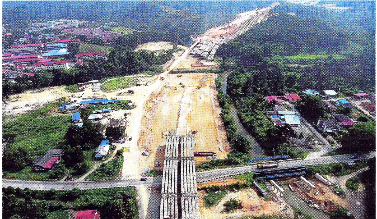
An East Coast Rail Link project construction site in Bentong, Pahang. ECRL will pass through five states and Putrajaya under the new deal. FILE PIC
