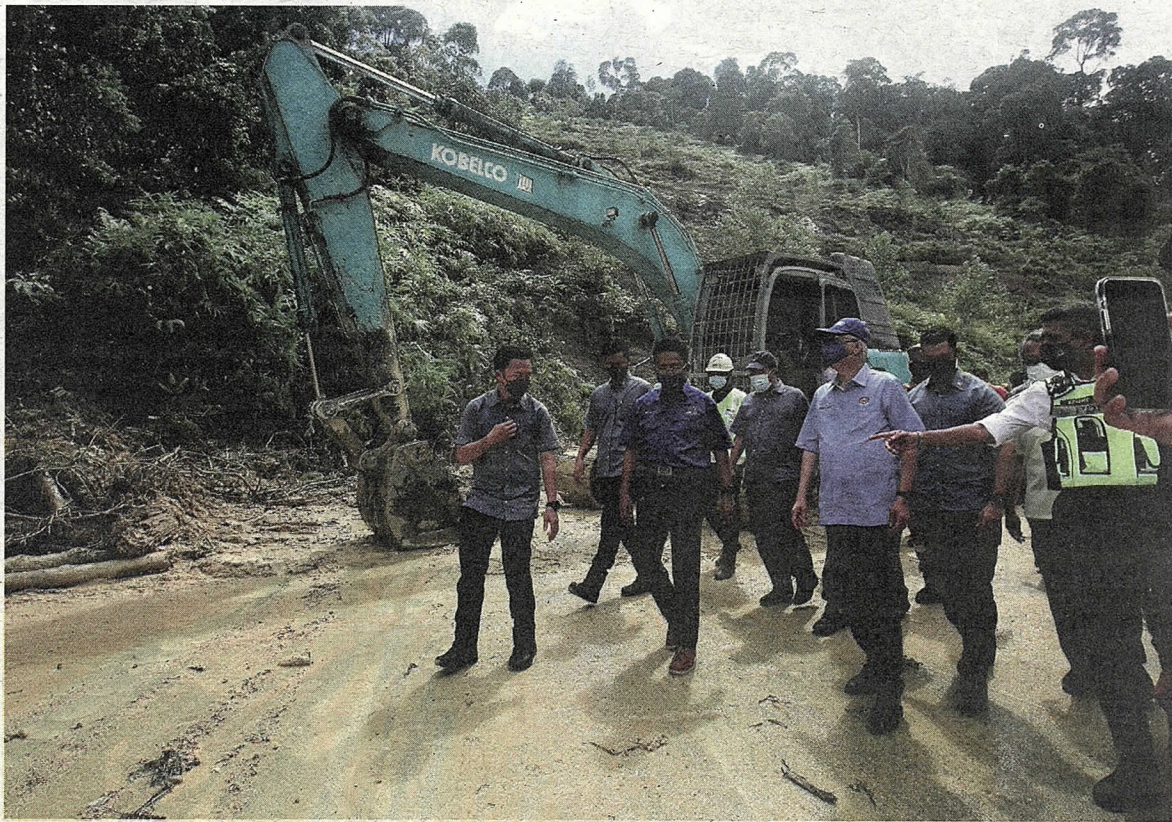
On the ground: Ismail Sabri surveying the damage caused by a landslide in Bukit Tangga, which is the main access to Jalan Seremban-Simpang Pertang connecting Jalan Pantai and Jeram Toi in Seremban. — Bernama
