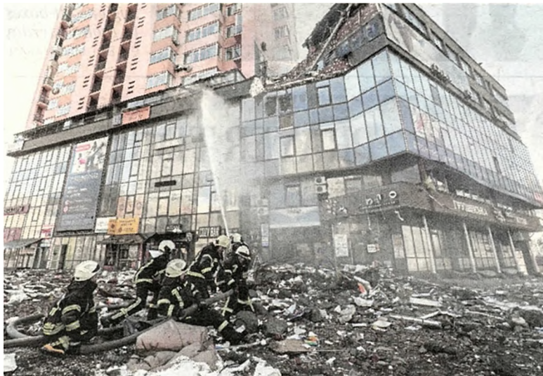
Ukrainian firefighters putting out a blaze at a high-rise apartment block, which was hit by shelling in Kyiv, yesterday. EPA PIC
