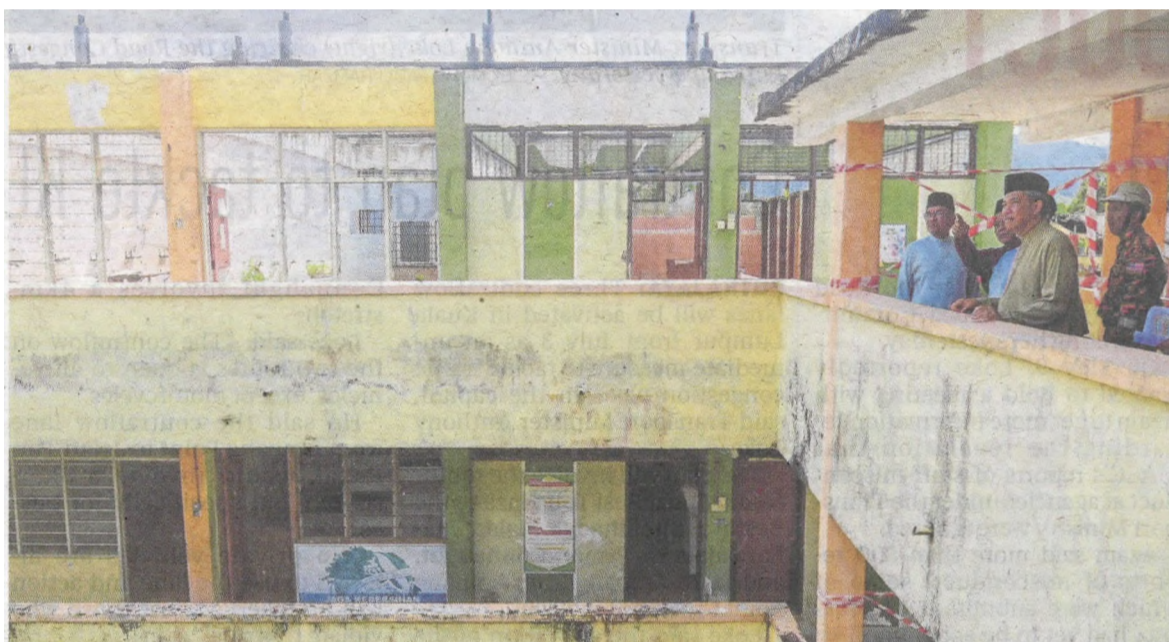
Prime Minister Datuk Seri Anwar Ibrahim (left) and Defence Minister Datuk Seri Mohamad Hasan (second from right) inspecting the boys' dormitory of SMKA Dato Haji Hassan Sail Pedas in Rembau yesterday. The boys' dormitory was damaged in a fire in July last year. BERNAMA PIC
