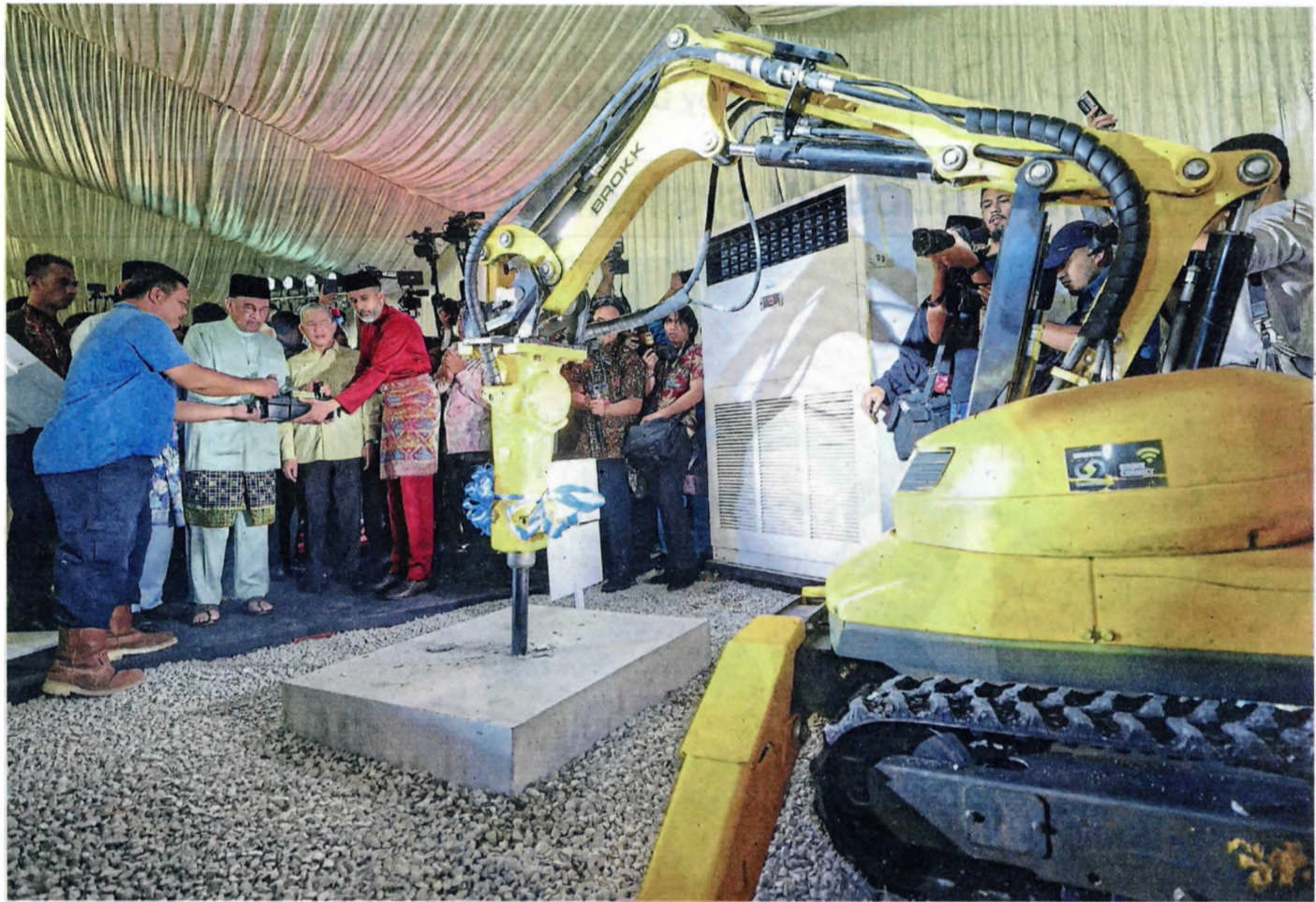
Symbolic start: Anwar officiating the groundbreaking ceremony of Masjid Madani in Kuala Lumpur. — Bernama
