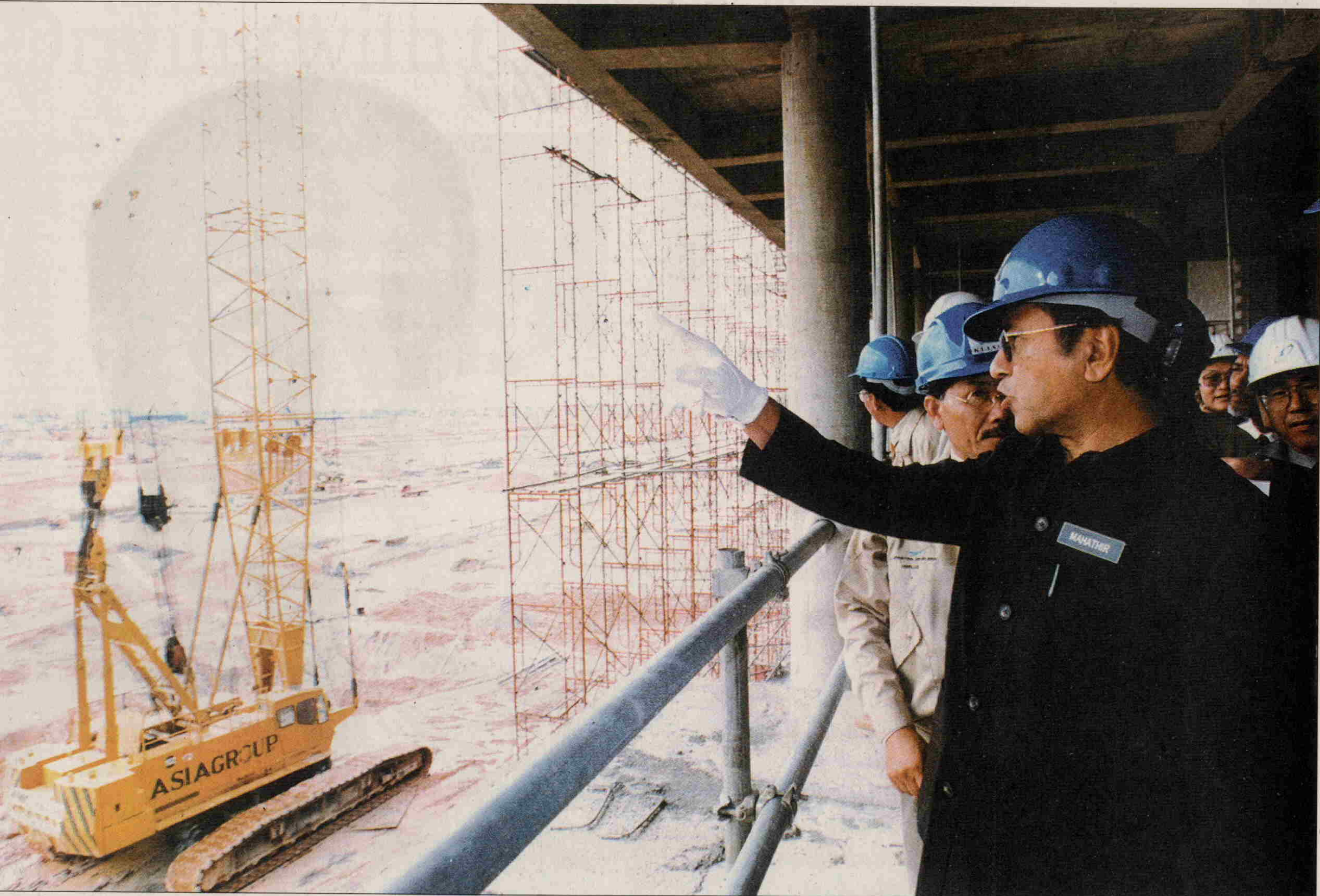
NATION'S PRIDE: Dr Mahathir checking on the progress of work on Kuala Lumpur International Airport in Sepang in 1996
